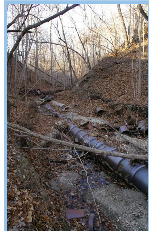
Exposed water use line
